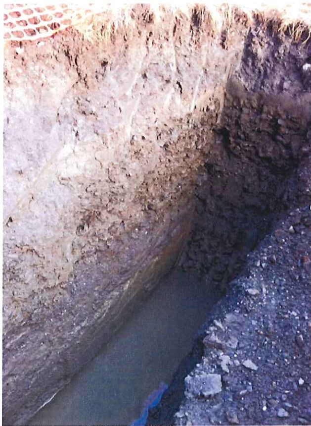
Test Pit DT-3, Note Standing Water & Clay Soil Layer
