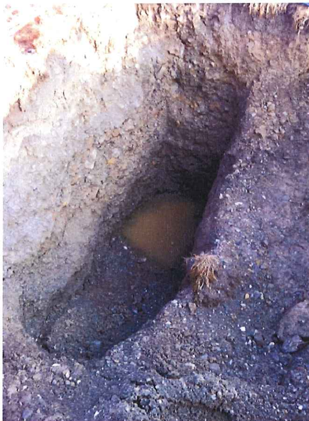
Test Pit DT-2, Note Standing Water
